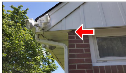
2.0 Item 2(Picture) Example/ Sample- right side of home – gap/ opening
