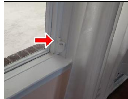
3.6 Item 4(Picture) Example/ Sample- Living Room window missing handle (these windows were not operated)
