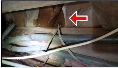
5.3 Item 6(Picture) Example/ Sample- near rear of home –wet area suspected plumbing leak
