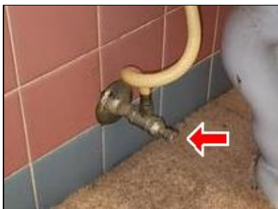
5.3 Item 1(Picture) Example/ Sample- Primary Bathroom- water cutoff handle missing
