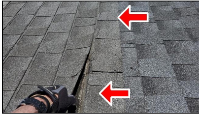
1.0 Item 10(Picture) Example/ Sample- rear of home shingle damaged, improper installation
