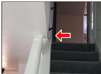
3.4 Item 1(Picture) Example/ Sample- does not return to the wall
