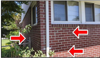
2.0 Item 9(Picture) Example/ Sample- right side of home and rear – cracking
