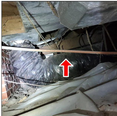
5.3 Item 10(Picture) Example/ Sample- near the front – plumbing pipe inadequate support
