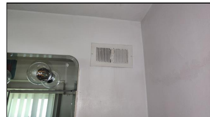
7.0 Item 3(Picture) Example/ Sample- Primary Bathroom- HVAC supply did not produced condition air when tested
