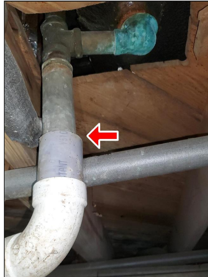
5.3 Item 8(Picture) Example/ Sample- near the front of the home –pipe connection improper leaks will probably occur
