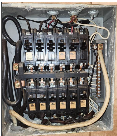
6.3 Item 2(Picture) Electrical sub panel uncovered by inspector during inspection located in kitchen closet
