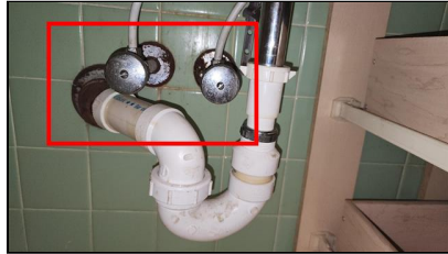
5.4 Item 1(Picture) Example/ Sample- Hall Bathroom Sink
