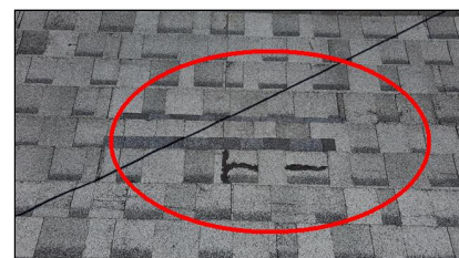
1.0 Item 9(Picture) Example/ Sample- rear of home – substandard installation/repairs
