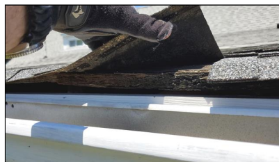
1.0 Item 5(Picture) Example/ Sample- rear of home – screened in porch area –exposed sheathing component(s) - deterioration
