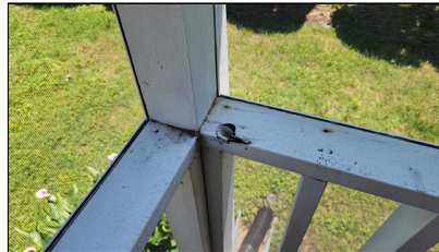
2.0 Item 14(Picture) Example/ Sample- deterioration
