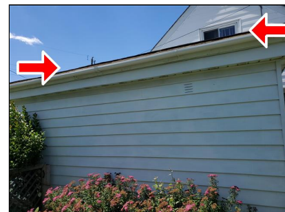
1.0 Item 3(Picture) Example/ Sample- left side of home carport area – exposed sheathing components, sheathing deterioration
