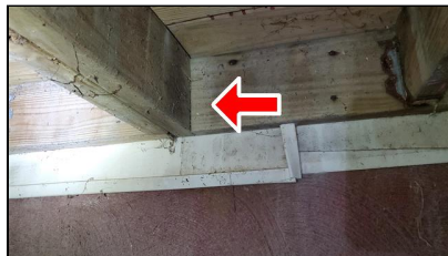
2.1 Item 6(Picture) Example/ Sample- floor joist not properly supported at ends – just nails considered insufficient
