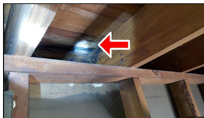
1.0 Item 4(Picture) Example/ Sample- shed at the carport area – roof sheathing deteriorated
