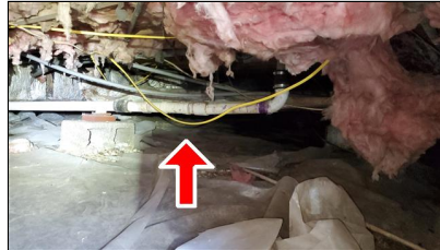
6.5 Item 8(Picture) Example/ Sample- loose wire – crawlspace near rear of home
