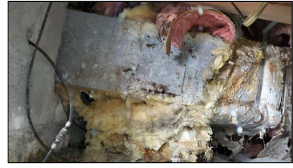
7.5 Item 3(Picture) Example/ Sample- damaged insulation
