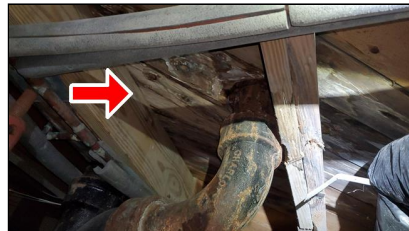
5.3 Item 11(Picture) Example/ Sample- near the front of home – active leak
