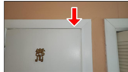
3.3 Item 3(Picture) Example/ Sample- Rear Right Bedroom- Rubs the jamb
