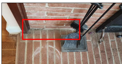
7.7 Item 2(Picture) Example/ Sample- hearth separation/ cracking
