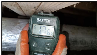
4.0 Item 1(Picture) elevated wood moisture content(WMC) 17.6% +/- addition crawlspace
