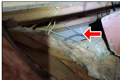
5.3 Item 3(Picture) Example/ Sample- addition crawlspace –plumbing pipe Inadequate support
