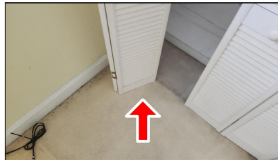
3.3 Item 2(Picture) Example/ Sample- Rear Left Bedroom Closet- Rubs the floor
