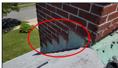
1.0 Item 7(Picture) Example/ Sample- rusted flashings
