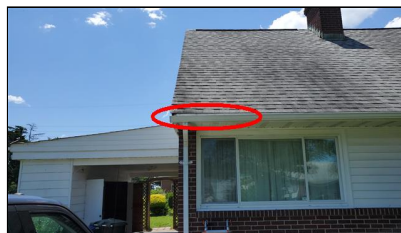
1.0 Item 2(Picture) Example/ Sample- Front of home- exposed sheathing component(s)
