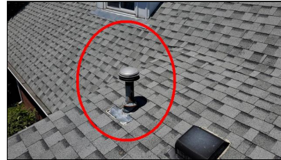
7.6 Item 2(Picture) gas vent termination clearance requirement to windows for example considered improper
