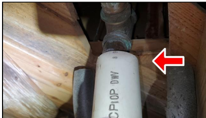
5.3 Item 9(Picture) Example/ Sample- near the front of the home –pipe connection improper leaks will probably occur
