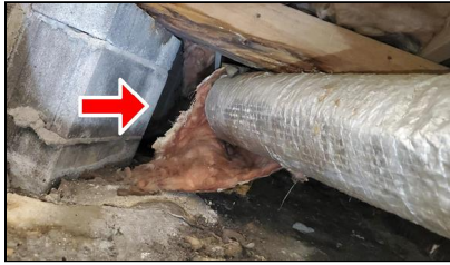
7.5 Item 1(Picture) Example/ Sample- addition crawlspace – insulation damaged
