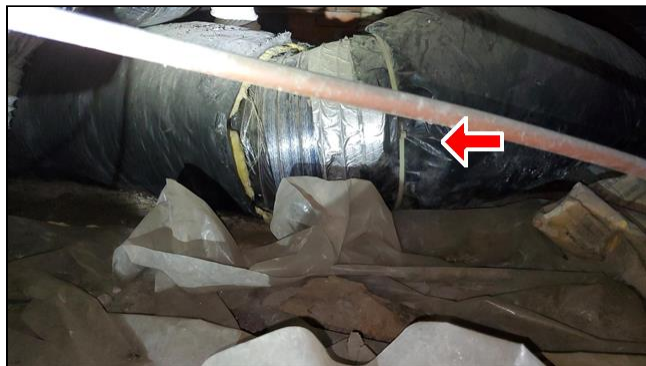
7.5 Item 6(Picture) Example/Sample- near front of home – insulation missing
