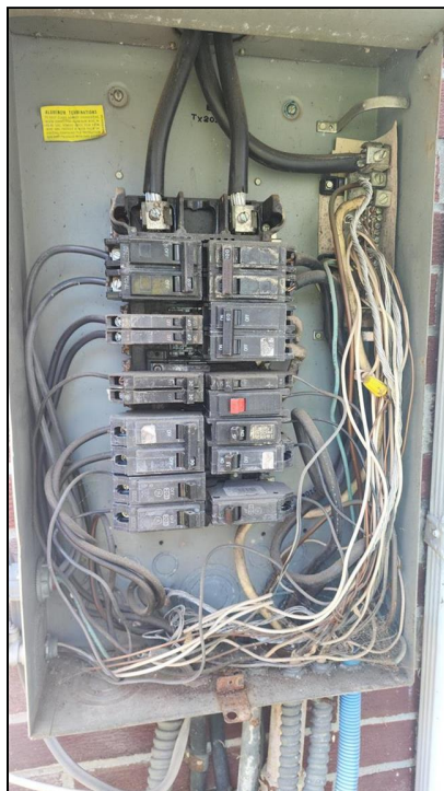
6.3 Item 1(Picture) Electrical panel uncovered by inspector during inspection located at rear of home
