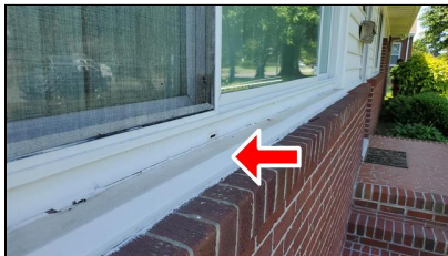
2.0 Item 16(Picture) Example/ Sample- substandard installation such as –Sill slope improper
