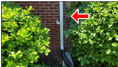
1.1 Item 1(Picture) Example/ Sample- front of home – downspout loose
