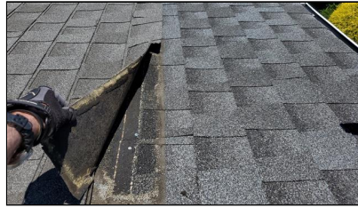
1.0 Item 11(Picture) Example/ Sample- rear of home – improper installation, damage
