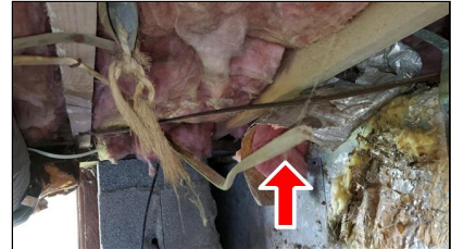
6.5 Item 9(Picture) Example/ Sample- near the rear – wire not properly terminated
