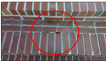
2.1 Item 1(Picture) Example/ Sample- front of home –deteriorating and/or missing mortar
