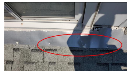
1.0 Item 6(Picture) Example/ Sample- rear of home – sealant maintenance for nail heads required
