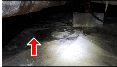
4.0 Item 5(Picture) Example/ Sample- rear of home – wet/water and possible contaminated conditions which is considered a health hazard
