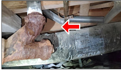
5.3 Item 7(Picture) Example/ Sample- near the front of the home – active leak, cast-iron pipe and galvanized pipe corrosion
