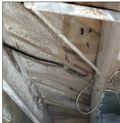
4.0 Item 3(Picture) Example/ Sample- fungi on wood member(s)
