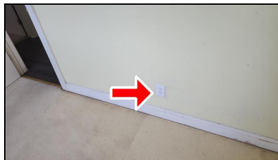
6.6 Item 1(Picture) Example/ Sample- Rear Left Bedroom- Loose outlet
