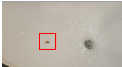
5.4 Item 11(Picture) Example/ Sample- Second level Bathroom Shower- tub damage/ rusted
