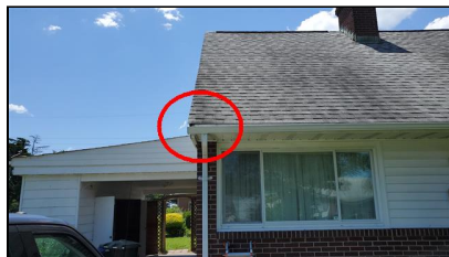
2.0 Item 1(Picture) Example/ Sample- Front of home- wood component(s) deteriorated and/or appear to be
