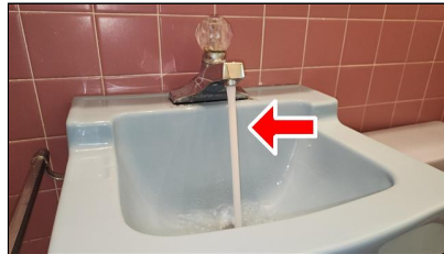
5.4 Item 8(Picture) Example/ Sample- Primary Bathroom Sink- sink drain does not keep up with the water flow
