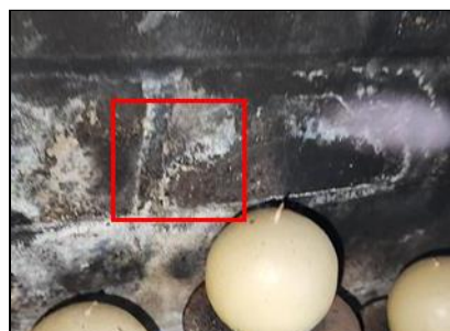
7.7 Item 1(Picture) Example/ Sample- firebox deteriorated and/ or cracked
