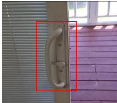
3.3 Item 1(Picture) Example/ Sample- Rear Door- Loose door handle/locking handles
