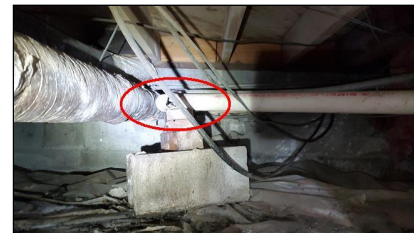
5.3 Item 5(Picture) Example/ Sample- rear of home – active waste pipe leak and damaged pipe
