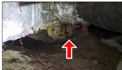
7.5 Item 9(Picture) Example/Sample- near the middle damaged insulation
