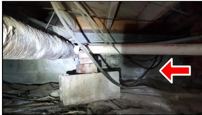
6.5 Item 10(Picture) Example/ Sample- rear of home loose wires
