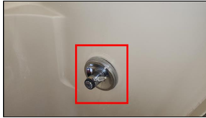
5.4 Item 4(Picture) Example/ Sample- Laundry Room Shower- plumbing tree component is loose
