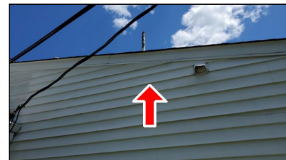
2.0 Item 3(Picture) Example/ Sample- rear of home – siding loose
