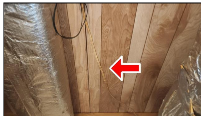
6.6 Item 2(Picture) Example/ Sample- Kitchen Closet- Loose electrical wire (not properly secured)
