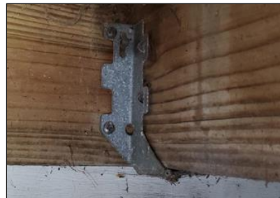
2.1 Item 7(Picture) Example/ Sample- improper fasteners used in joist hangers
