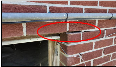
2.0 Item 12(Picture) Example/ Sample- rear of home mortar missing
