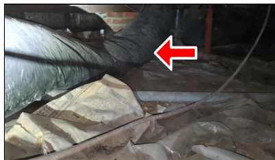
7.5 Item 7(Picture) Example/Sample- new front of home ducting damaged, inadequate support
