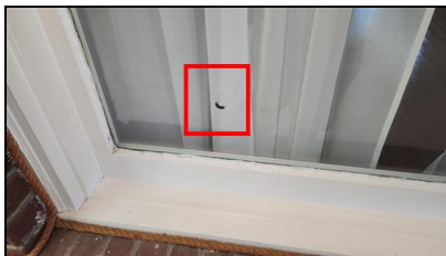
3.6 Item 5(Picture) Example/ Sample- Rear Den/Living Room- Damaged glazing/glass
