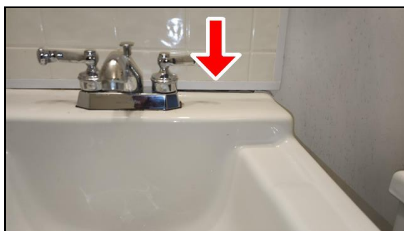
3.0 Item 19(Picture) Example/ Sample- Second level Bathroom Sink
