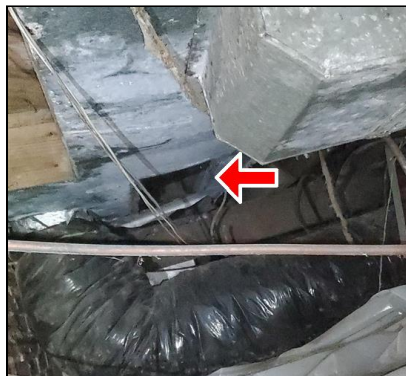
7.5 Item 8(Picture) Example/Sample- near the front of the home – possible opening to ducting system
