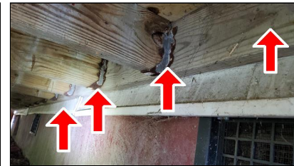
2.1 Item 5(Picture) Example/ Sample- rusted hangers, ledger board improperly secured to structure
