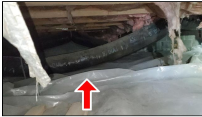
7.5 Item 4(Picture) Example/ Sample- near the front – inadequate support
