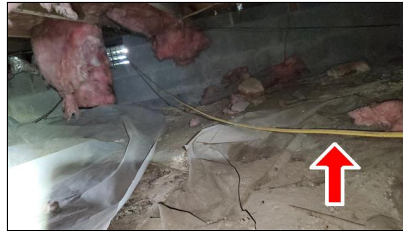
6.5 Item 11(Picture) Example/ Sample- front of home – loose wire
