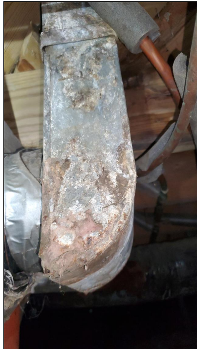
7.5 Item 5(Picture) Example/ Sample- front of home – deterioration, missing insulation
